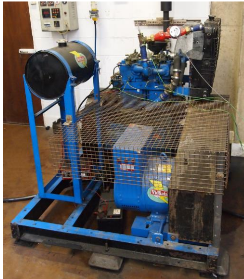
Figure 3.3 Lister CS diesel Engine and Generator
