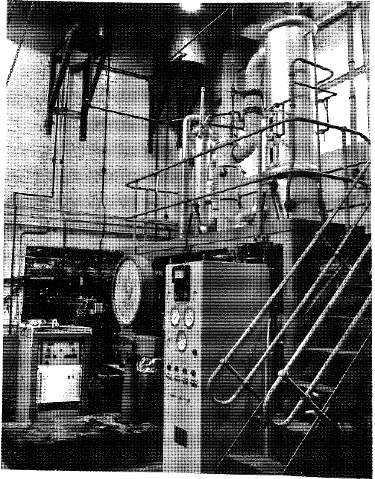
Photograph showing the double effect evaporator with the MDP. 200 Remote cabinet in the left background.
