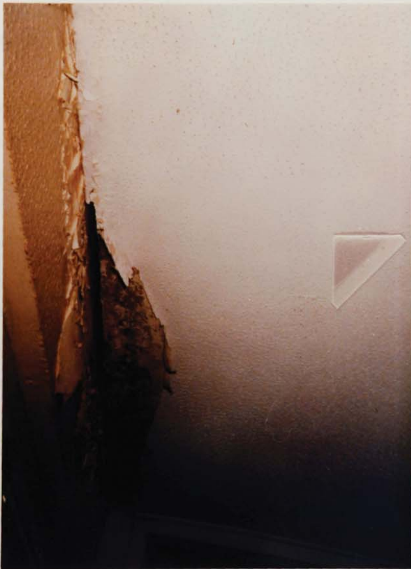
Plate 8-3 The joint between floor units and external load bearing panels Lapworth House.
