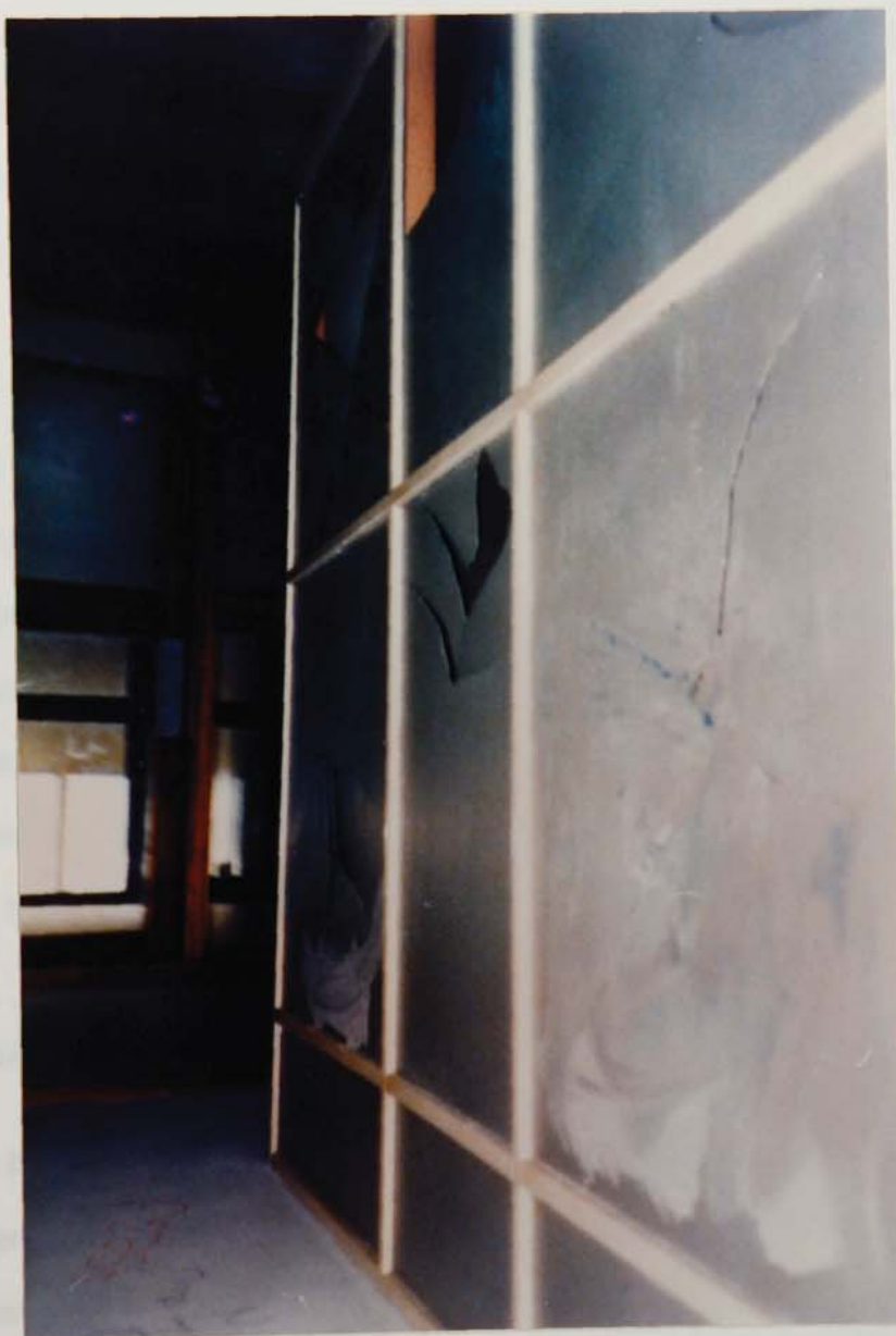
Plate 8-8 The damaged partitions in Netley House block
