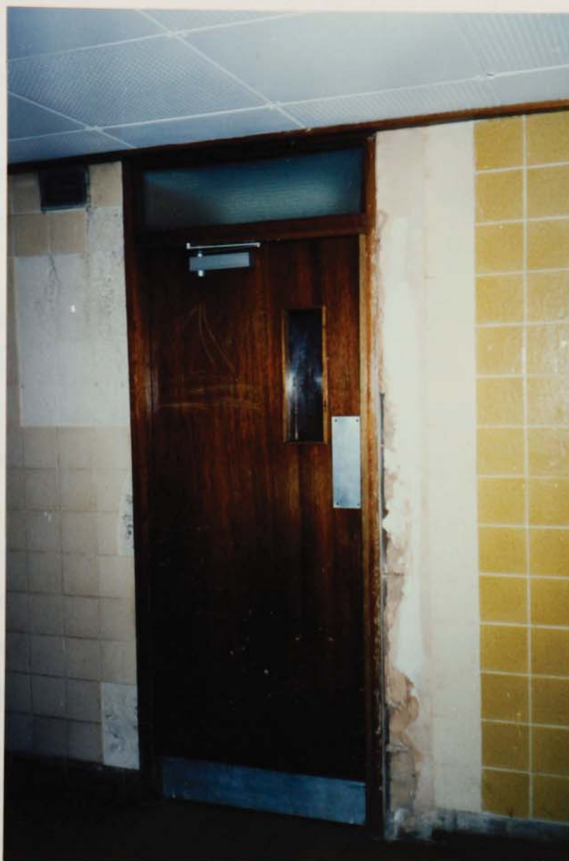
Plate 8-1 The damaged back door in the Normansell Tower
