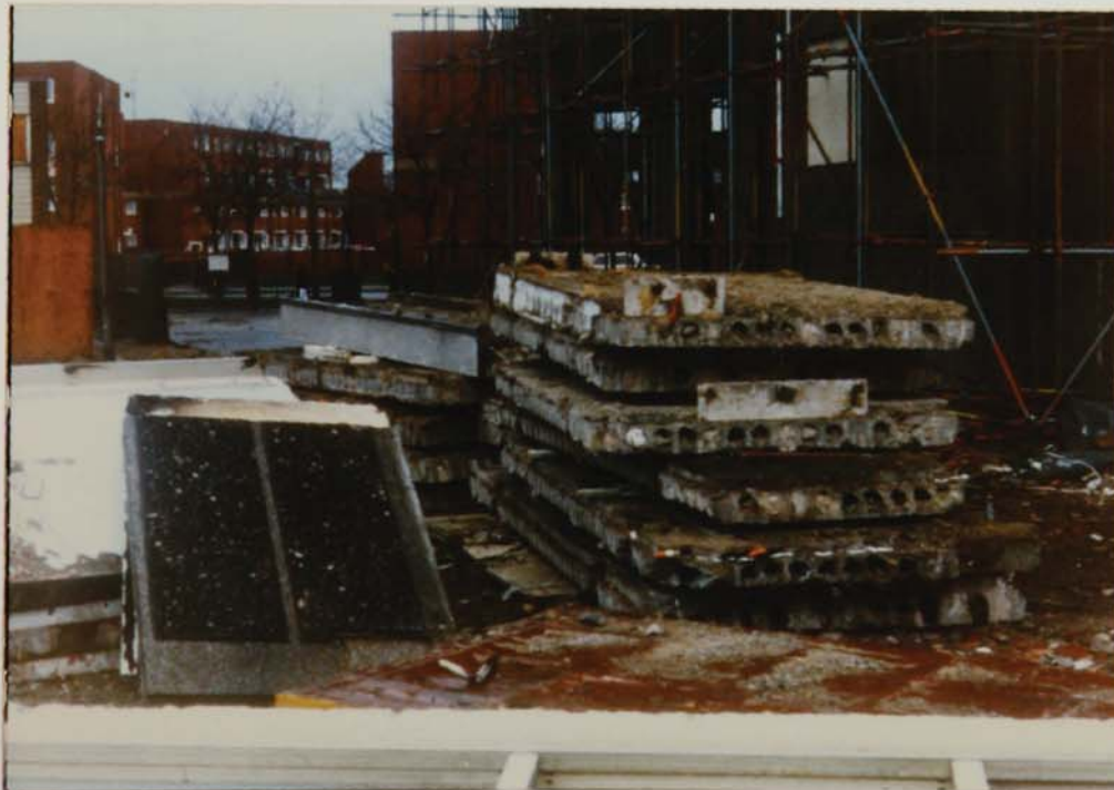
plate 9-2 The dismsantled floor panels of Ronan Point
