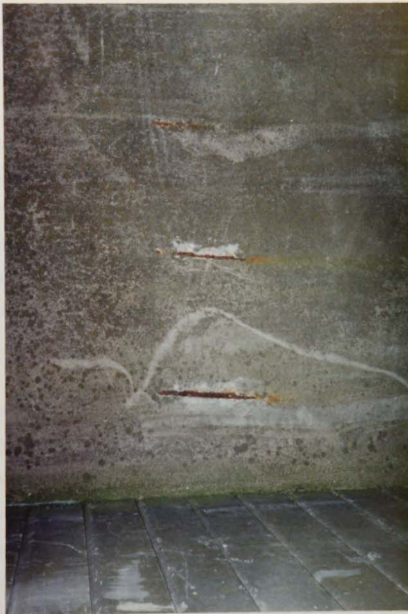
Plate 8-5 Exposed reinforcement bar in the parapet of Woburn House
