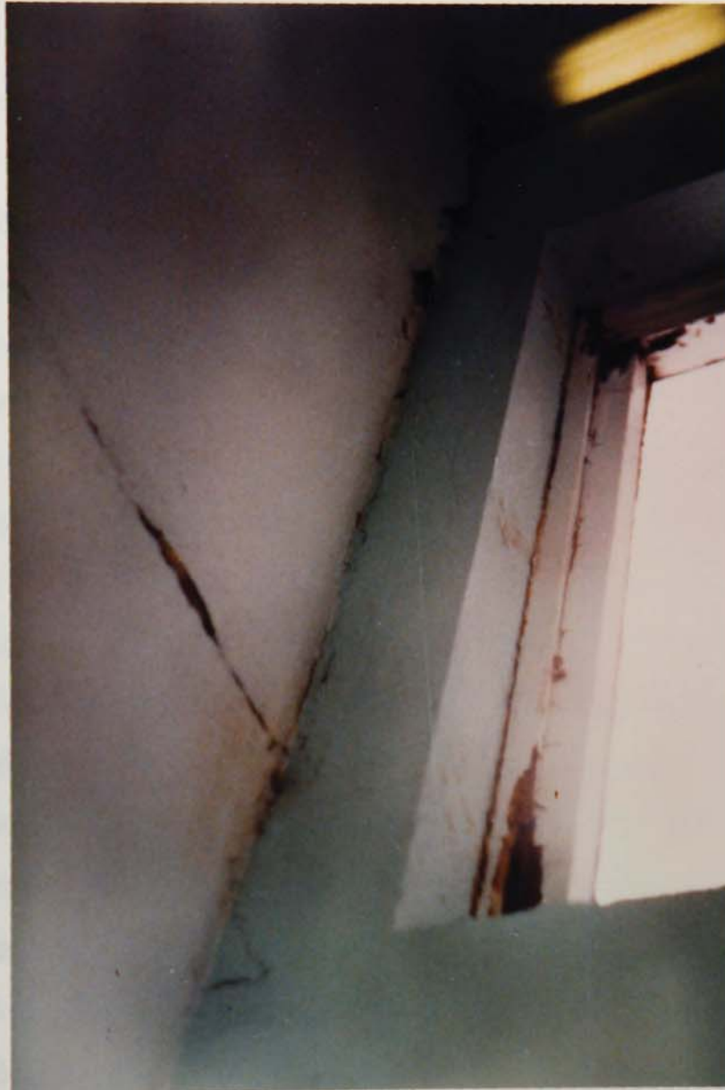
Plate 5-1 Structural connection and external fixture defects
