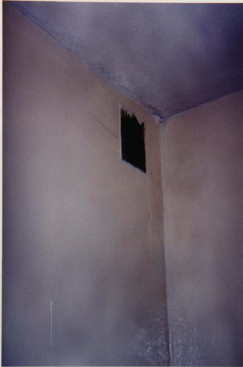
Plate 8-2 Mould layer covered the ventilation duct openings in the Stokesay House roof
